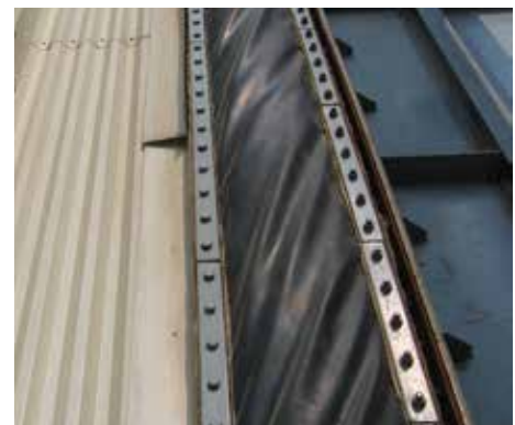
Fluastal exposed to lateral movement in horizontal duct.
