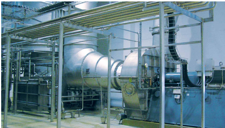
Fan installed in vapour compression plant Photo: Piller Blower & Compressors GmbH
