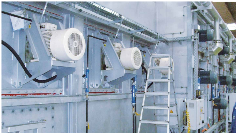
Continuous kilns' fan drives for the heat treatment of metal strips Photo by courtesy of Aurubis AG
